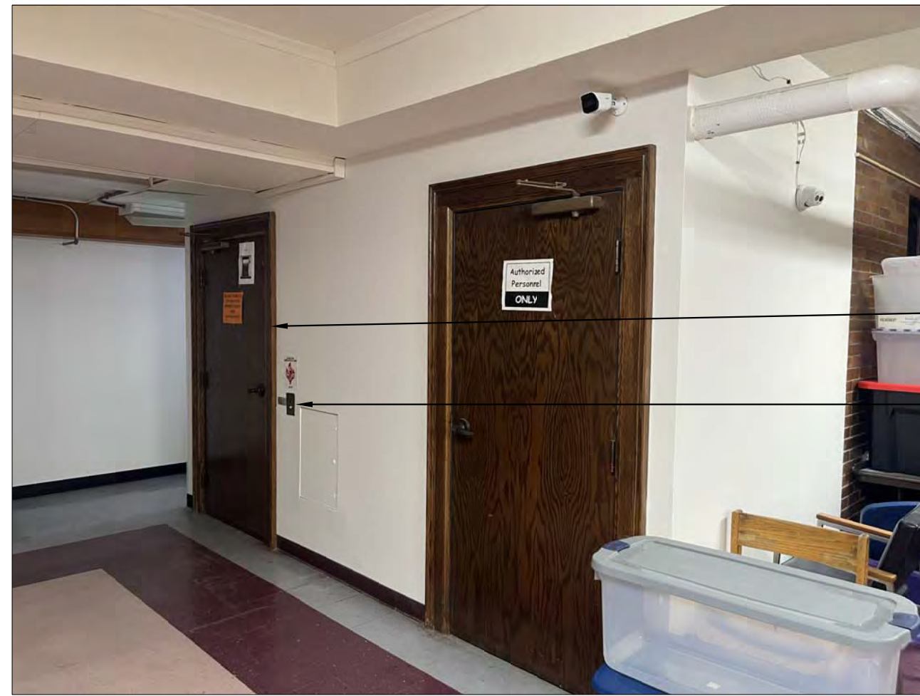
1 LOWER LEVEL DOORS / TRIM WORK AT LIFT & MACHINE RM A5 NO SCALE
