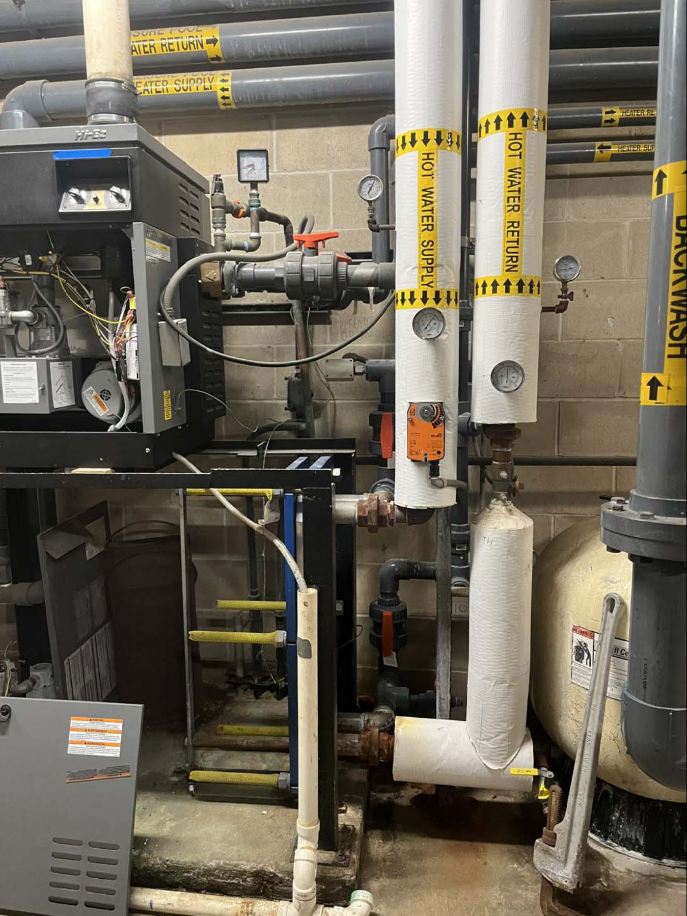
5 Existing Therapy Pool 2019 Install Example - Leisure/Whirlpool to match Therapy H200 not to scale
