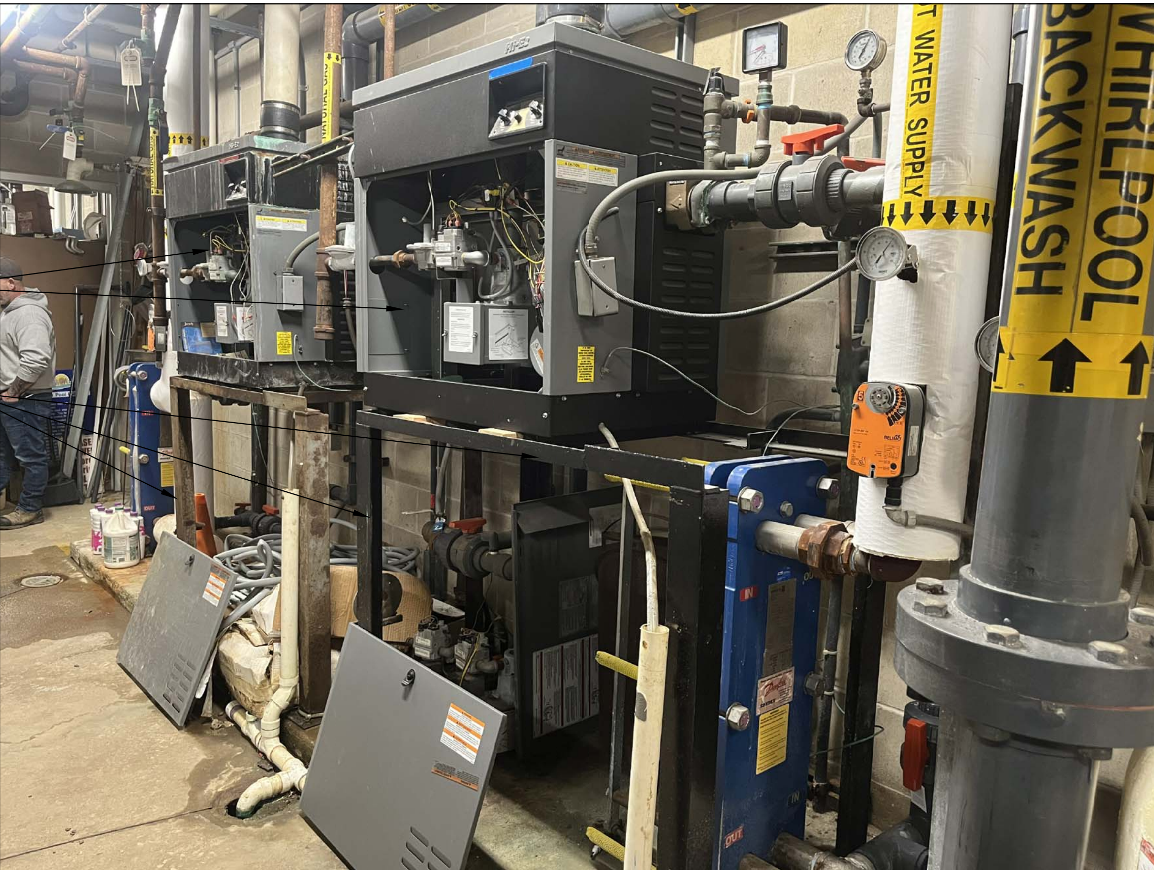
4 Current Image of Existing Heat Exchangers / Heater Conditions For Reference Only H200 not to scale
